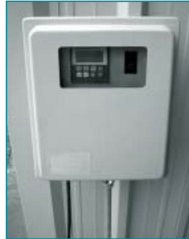
Flow Monitoring System
