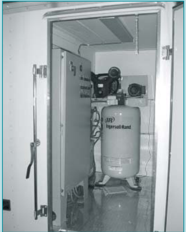
Control panel mounted in a separate partitioned room.
